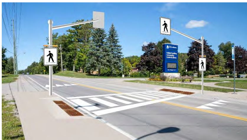
Figure 2 Yonge Street adjacent to Holland Landing Community Centre in the Town of East Gwillimbury
